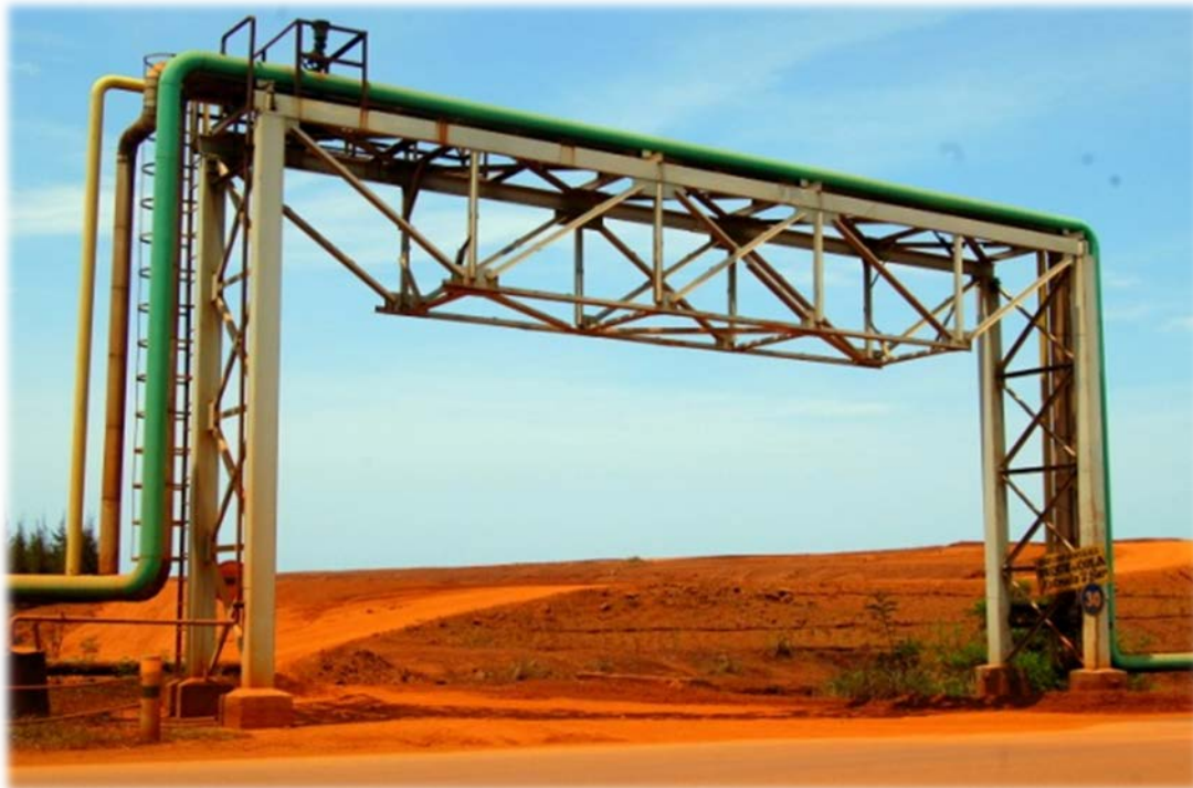
Pipelines on the bayside of the road
